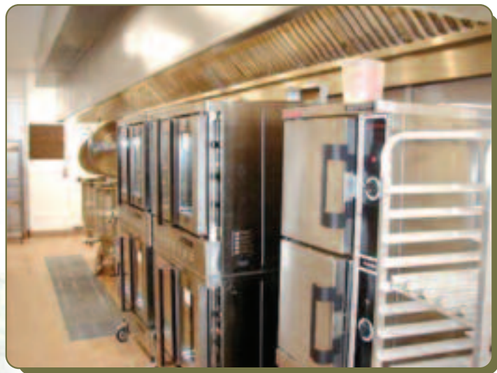
Typical Ventilator Installation - University of Maine - Orono, ME
